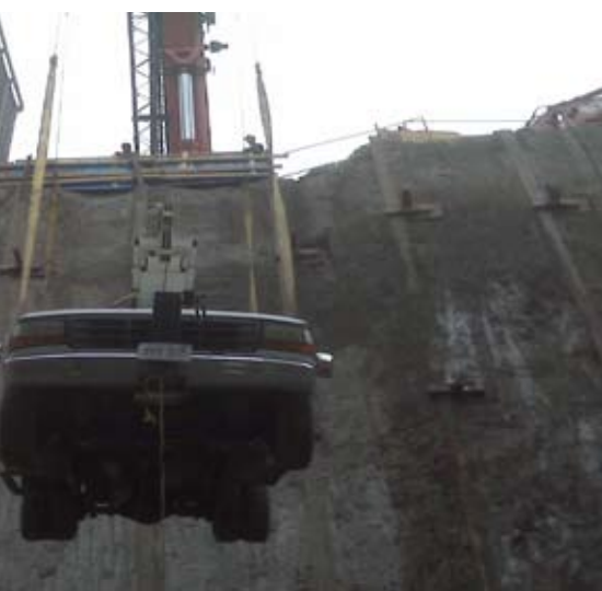
Nothing appears impossible for Fred Constable & Son Ltd. This job required drilling some extra wells in the bottom of a completed excavation with about a 60' drop from the road. The building in the background is the ManuLife centre, downtown Toronto.
